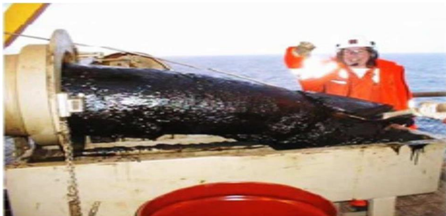
Figure.1. Wax deposition plug in the wellbore on platform C in the North Sea (Theyab et al, 2018).
